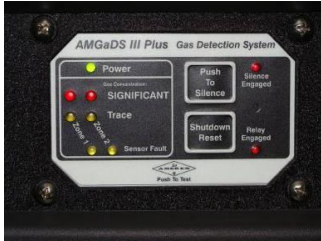
Gas Detection System
